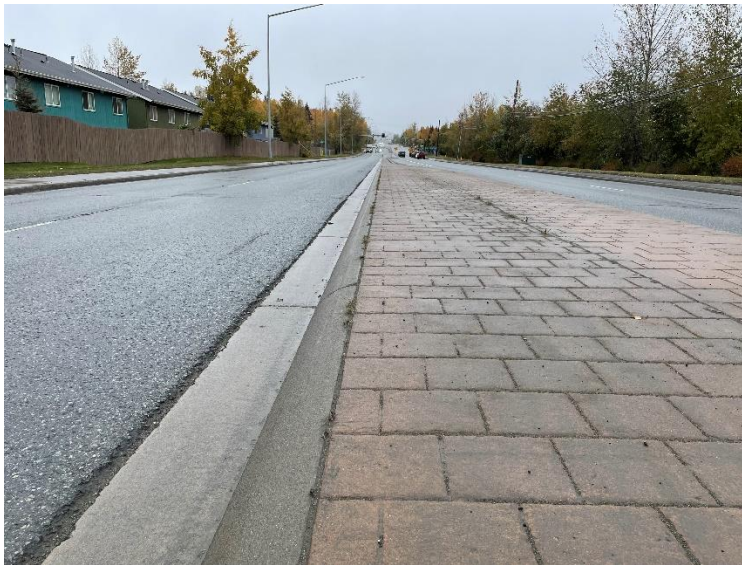
Figure 6.4 – Muldoon Rd after sweeping operations.
